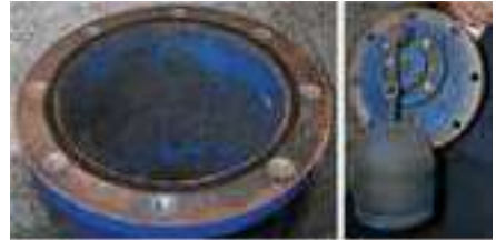
Figure 4 – Sludge build-up on fusion bonded epoxy coated internal valve casting.
