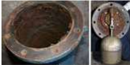
Figure 2 – Sludge build-up on uncoated internal valve casting.
