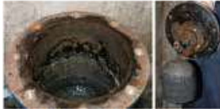
Figure 3 – Sludge build-up on two-part epoxy coated internal valve casting.
